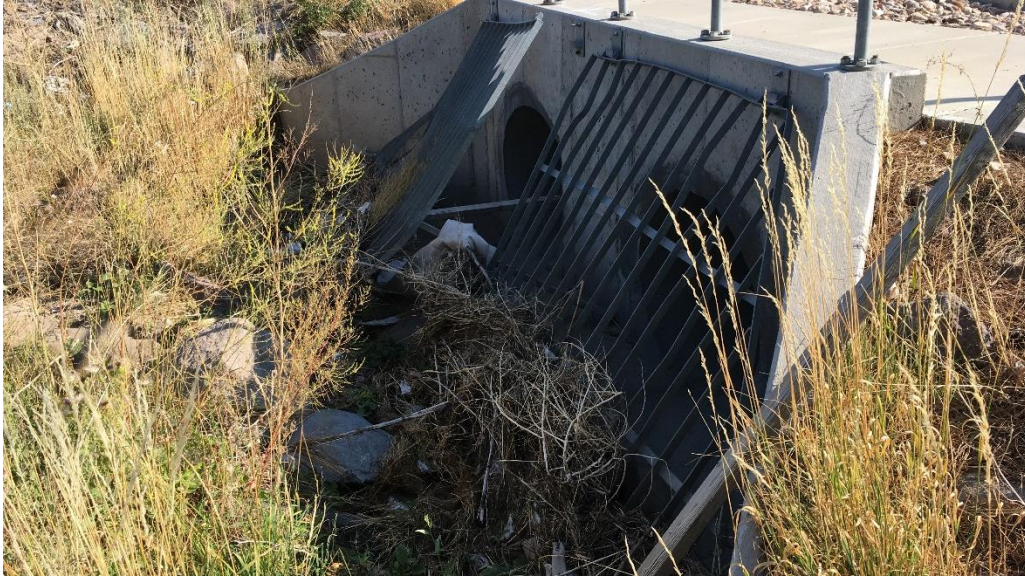
Photo 2-6: Example of a Trash Rack on Barneys Creek at Airport Rd
