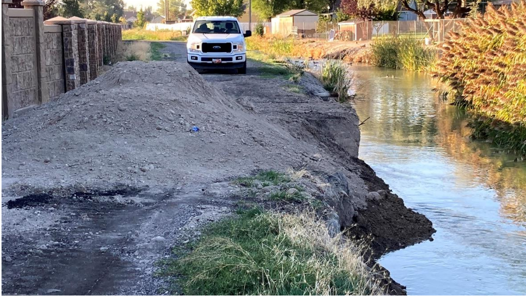
Photo 2-7: Recently Sloughed South Jordan Canal
