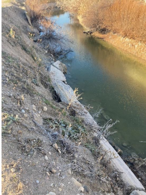
Photo 2-9: Example of Eroding Bank Protection on Utah and Salt Lake Canal
