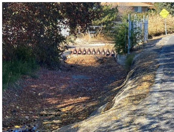
Photo 2-14: Trash Rack on South Jordan Canal
