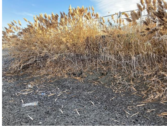
Photo 2-12: Excessive Vegetation Blocking the Storm Water Dumpout on USLC to Midas Creek
