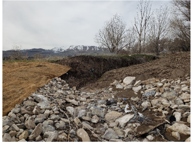
Channel erosion next to South Hills Middle School
