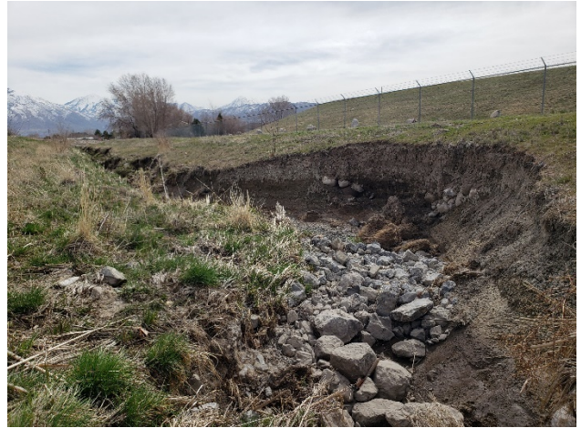
Channel erosion at approximately 3250 West
