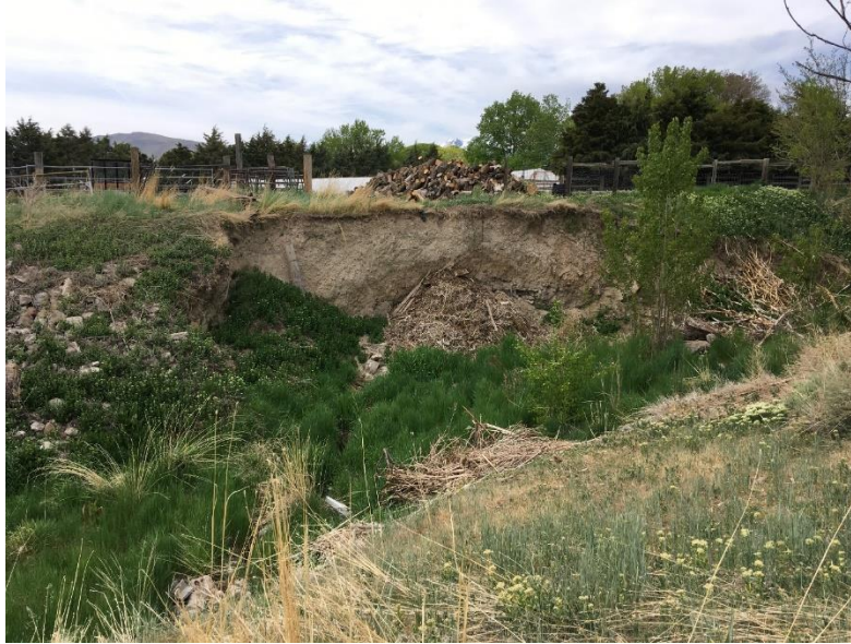
Photo 2-3 Bank Erosion Upstream of Bangerter Highway
