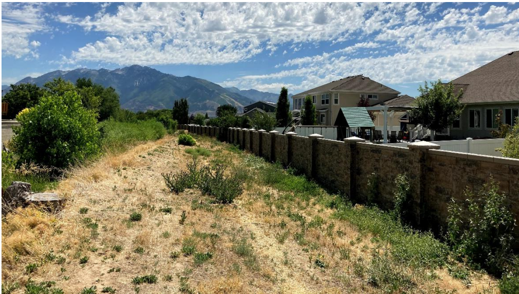
Photo 2-2 Portion of Uncertified Levee on Midas Creek Between 2700 West and the Utah and Salt Lake Canal
