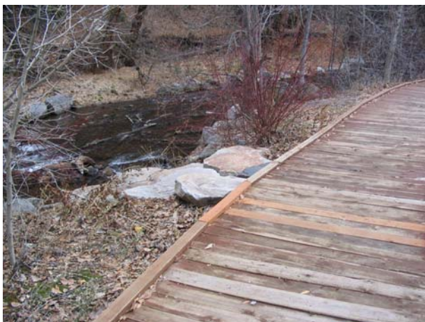
Figure 4.8 A successful bank stabilization project in a heavily used recreation site in Mill Creek Canyon that included natural rock steps to access the creek and a boardwalk to prevent vegetation trampling and erosion.
