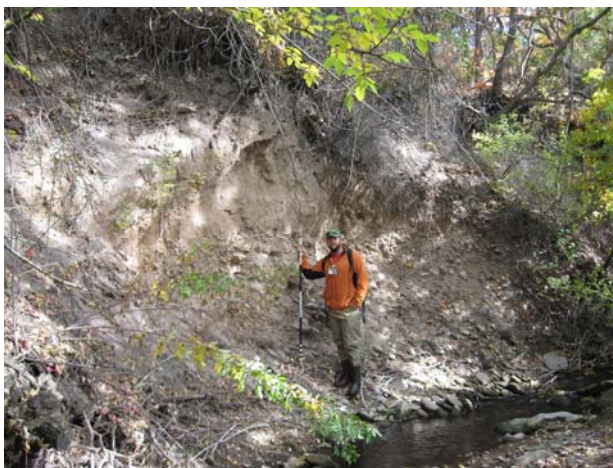
Figure 2.6 An Example of severe erosion on Lower Emigration Creek that is considered a “hotspot” on the Bank Stability Metric map.
