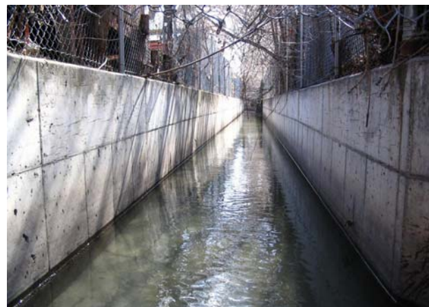
Several sections of concrete channel carry Mill Creek through residential and industrial areas.
