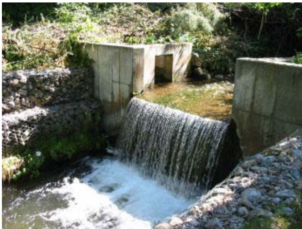
Historic diversion of Mill Creek (no longer used), Lower Mill Creek Sub-Watershed
