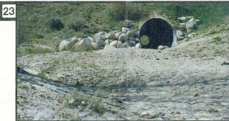
23 A) The build up of soil deposition east of 1300 East, 700 East and the landfill, is characteristic of Dry Creeks flow patterns. At these locations, the dimension of the floodplain is wide and riparian vegetation is sparse. B) The corrugation of the culvert pipe beneath 1300 East, does not provide a sure footing for trail users, especially equestrian users.
