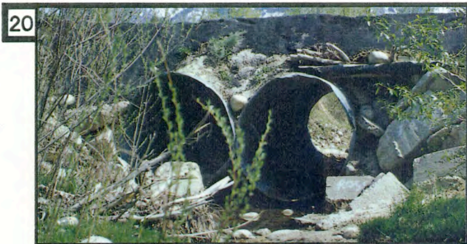
20 A) Stream flow velocities increase when passing through culverts. As flows exit culverts, increased streambank erosion occurs. B) Bridge structures rather than culverts, allow the stream to be more free flowing and will mitigate areas of streambank erosion caused by culvert structures.
