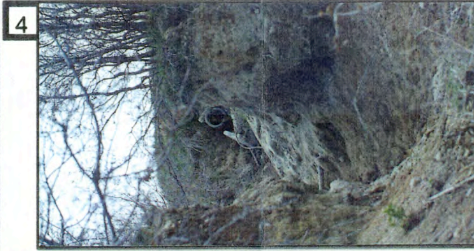
4 A) Storm water runoff was the cause of the severe wash out in this ravine. A storm sewer outlet designed to prevent soil erosion could have prevented this problem.
