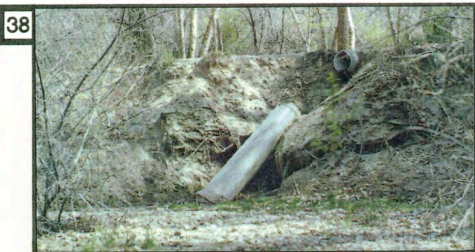
38 A) The location of this storm drainage outlet is closer to the streambed than most other outlets in the park. However, a lack of reinforcement to the streambank prevented the culvert from remaining stable. The streambank will continue to erode until reinforcement of the streambank takes place and a properly designed outlet is constructed.
