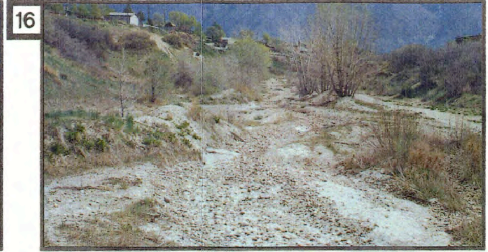
16 A) The modified alignment of Dry Creek in this specific area is unnatural in its appearance. Wide flood plains void of vegetation remain as a result of disturbances and stream alignment modifications. B) Vegetation communities in the area are water stressed.
