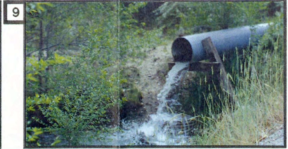
9 A) This outlet structure disposes of surplus irrigation water from the Sandy/Draper canal into Dry Creek. This structure is a good example of a properly designed culvert outlet that releases water into the Dry Creek streambed without damaging the environment. The erosive water forces are dissipated by locating a barrel filled with rocks beneath the outlet.
