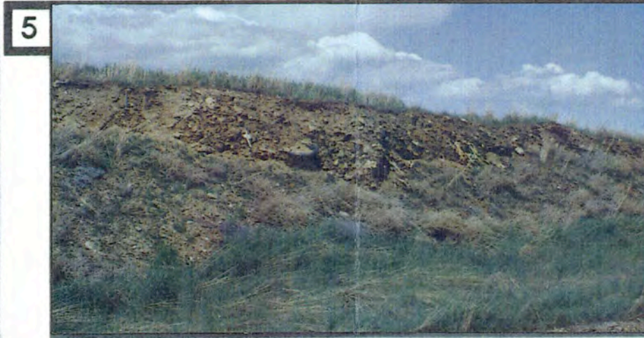
5 A) The proper closure of this inactive landfill is incomplete according to the standards for municipal solid waste landfills. Regulations which this landfill violate are: a sufficient protective layer of soil burying the refuse, surface water control, monitoring of methane gas, and establishment of a stable vegetation to prevent soil erosion. B) Ground stability for the construction of structures is considered to be poor on this site.
