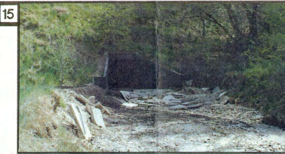
15 A) Historically, streambank protection at the outflow end of this culvert has involved the placement of concrete slabs. Although it is not the most attractive method in preventing streambank erosion, it is inexpensive and effective. B) Development of a safe trail leading into the culvert is critical. C) Vegetation on the slope of the 700 East roadway consists primarily of annual grasses and noxious weeds. Roadway slopes at 700 East and 1300 East should be included on future plans for native revegetation and erosion control.
