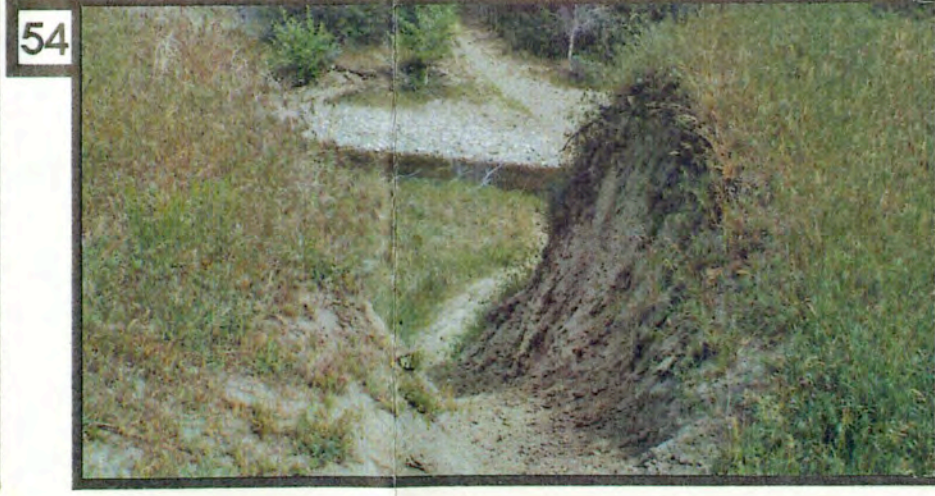
54 A) Trails similar to this one, contribute a large amount of sediment into Dry Creek unnecessarily. An equestrian/hiker trail crossing structure would be appropriate for trails creating this problem.
