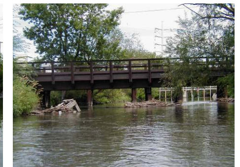
Figure 4.11.8 Two railroad bridges with debris (WP 12-10)
