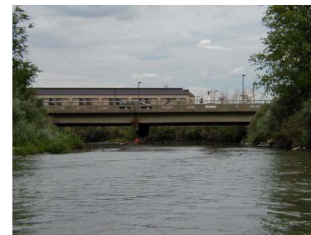
Figure 4.8.6 Flood debris at 4500 South bridge (WP 9-25)
