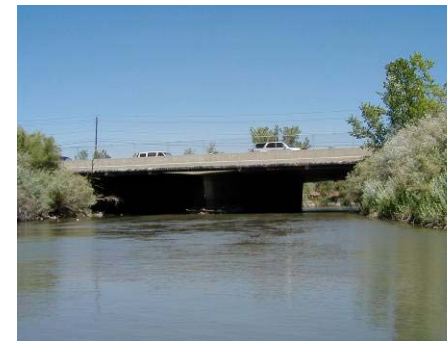
Figure 4.9.2 Vehicular bridge at 3300 South, built up debris (WP 10-05)
