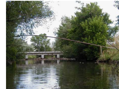
Figure 4.11.5 High pipeline (WP 12-07)
