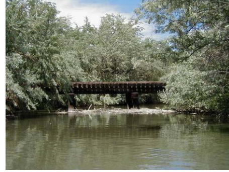
Figure 4.9.16 Debris collected at base of railroad bridge (WP 11-07)
