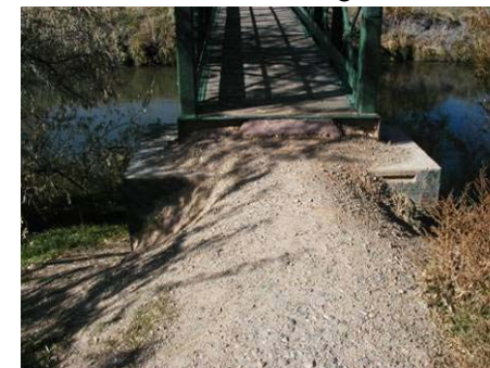
Figure 3.10.7 Non-accessible path to Bridge B18
