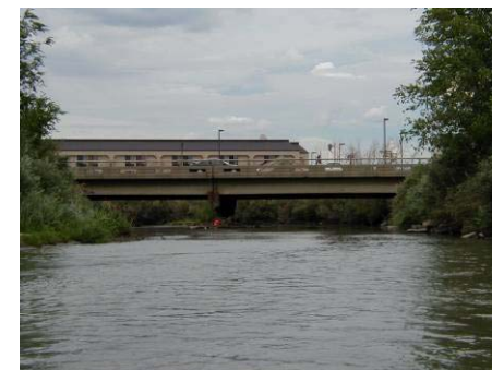
Figure 4.8.6 Flood debris at 4500 South bridge (WP 9-25)
