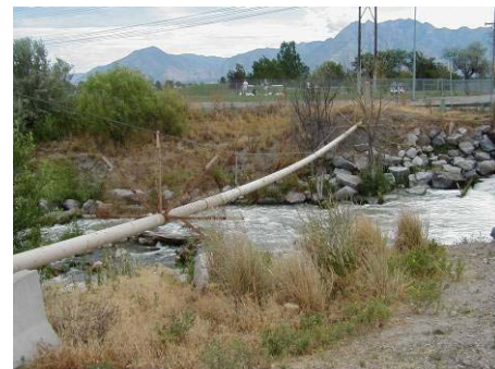
Figure 4.7.4 Qwest cable crossing river (WP 9-04)
