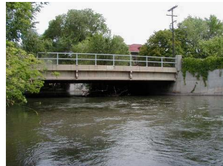
Figure 4.11.2 Low bridge at 200 South, debris (WP 12-04)
