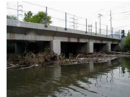
Figure 4.11.7 Flood debris at railroad bridge (WP 12-09)
