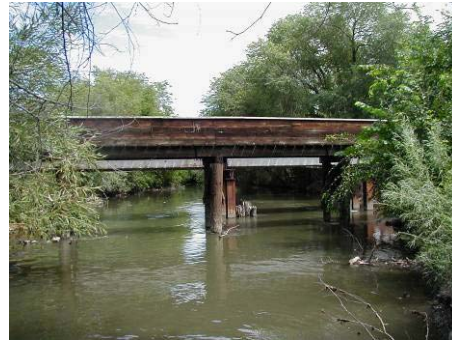
Figure 4.11.12 Railroad bridge near South Temple, debris (WP 12-14)
