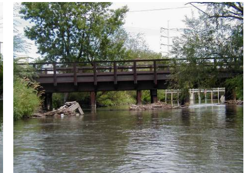
Figure 4.11.8 Two railroad bridges with debris (WP 12-10)
