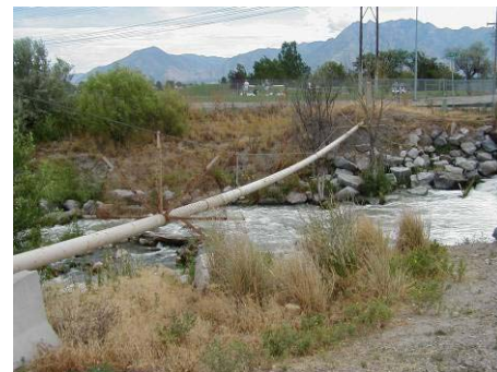
Figure 4.7.4 Qwest cable crossing river (WP 9-04)
