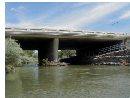
Figure 4.7.10 Vehicular bridge at 5400 South, flood debris (WP 9-14)
