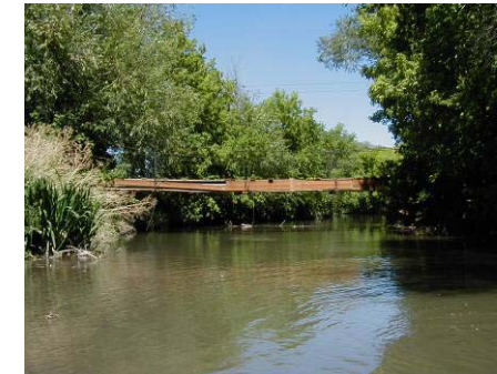
Figure 4.12.13 Pipeline covered with wood, cables hang down (WP 14-07)
