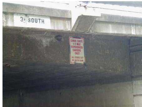
Figure 3.10.19 Warning sign on bridge, hard to notice (WP 11-32)
