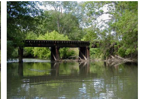
Figure 4.10.10 Railroad bridge at 900 South, debris covers half of channel (WP 11-22)
