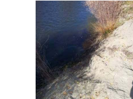
Figure 3.7.42 Washed out trail edge, west of Germania Park
