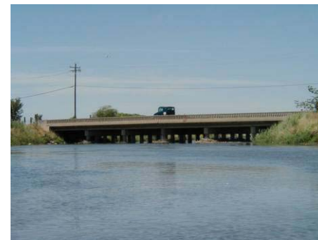
Figure 4.9.5 Woody debris in front of pillars (WP 10-11)
