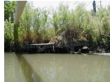
Figure 4.12.6 Abandoned boat launch near Redwood Road (WP 13-09)
