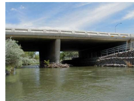
Figure 4.7.10 Vehicular bridge at 5400 South, flood debris (WP 9-14)
