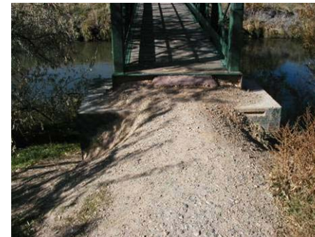
Figure 3.10.7 Non-accessible path to Bridge B18
