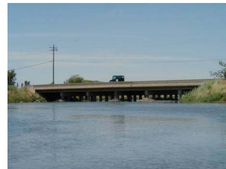
Figure 4.9.5 Woody debris in front of pillars (WP 10-11)
