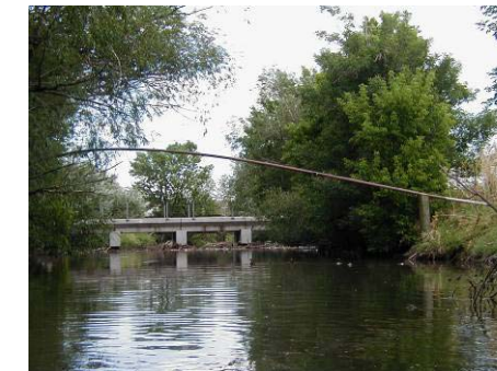
Figure 4.11.5 High pipeline (WP 12-07)
