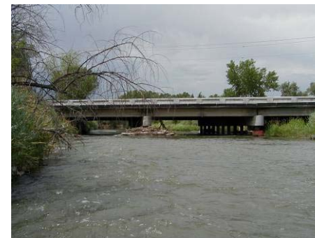
Figure 4.8.8 Flood debris at vehicular bridge at 3900 South (WP 9-30)
