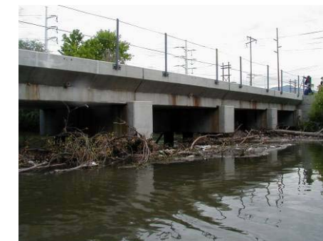
Figure 4.11.7 Flood debris at railroad bridge (WP 12-09)
