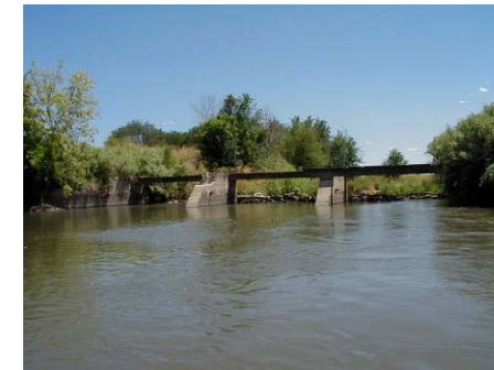
Figure 4.12.15 Historic irrigation dam, debris blocks entire channel (WP 14-09)
