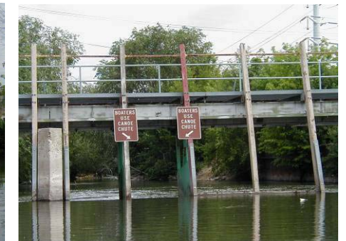
Figure 4.11.10 Warning sign for boaters (WP 12-12)
