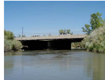
Figure 4.9.2 Vehicular bridge at 3300 South, built up debris (WP 10-05)
